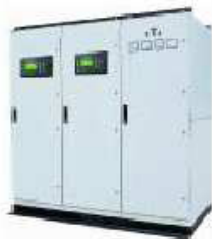
BGC Paralleling Control system
